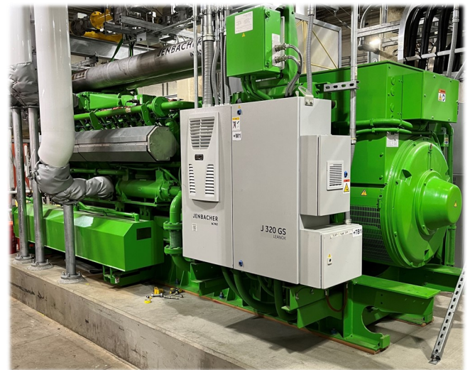
New Jenbacher cogeneration engine.
